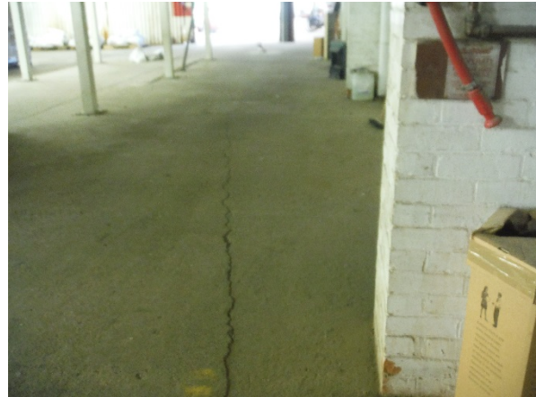
Photograph 4 – View of the crack damage to the floor slab to the south eastern part of the warehouse
