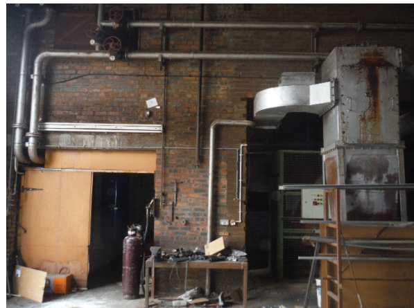
Photograph 6 – View of the HVAC unit
